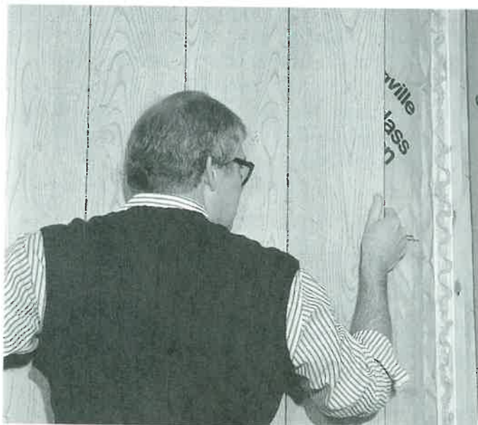
Figure 32-12. Prefinished plywood panels are attached with panel adhesive that has been applied to wall studs. (Franklin International)
