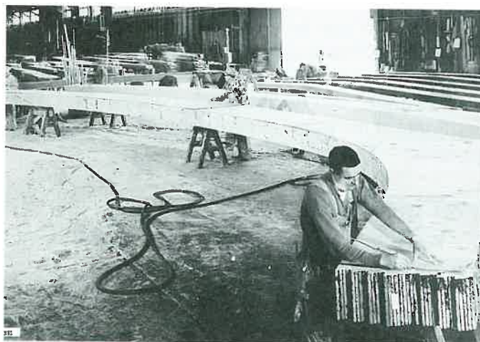
Figure 34-13. This lamination will be an arch for a cathedral ceiling. (Forest Products Laboratory)
