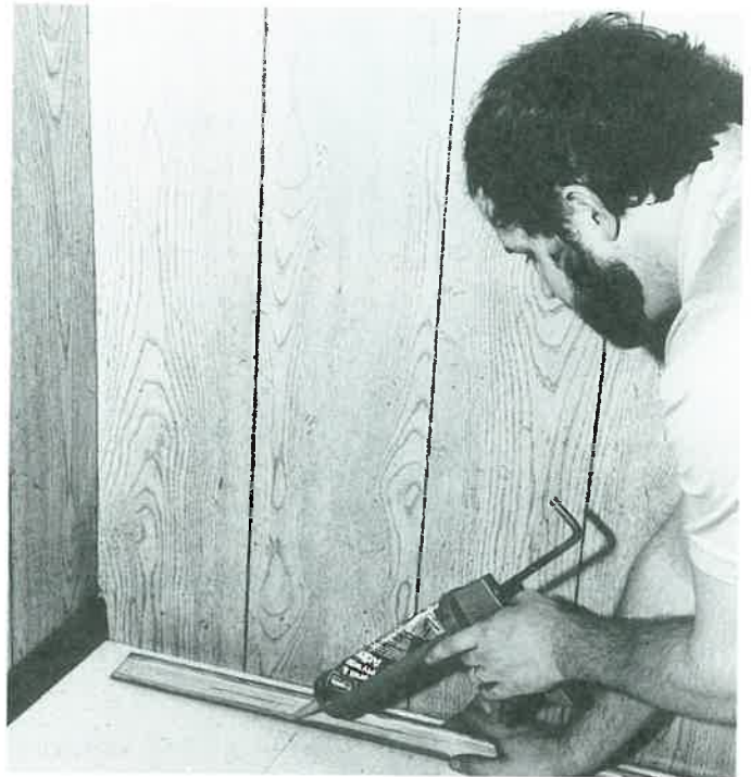
Figure 32-13. Install vinyl trim, base, and moldings with a vinyl adhesive. (Franklin International)
